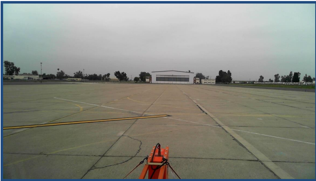
Figure F.39. CSA Terminal Representative Pavement Condition (Sta. 8+00)
