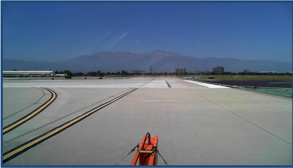
Figure F.8. Taxiway W Representative Pavement Condition (Sta. 1+50)
