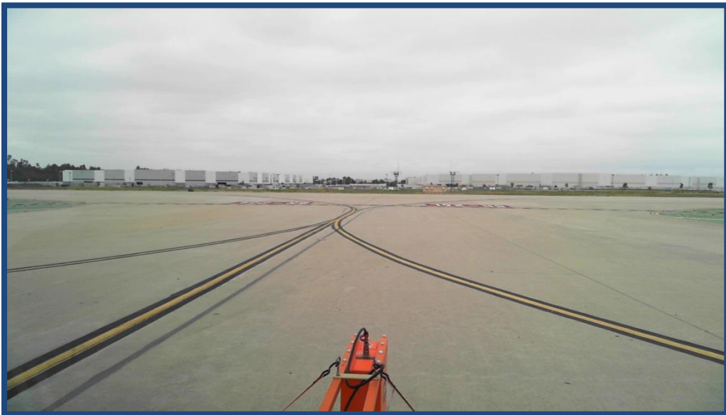
Figure F.25. Taxiway U Representative Pavement Condition (Sta. 2+75)
