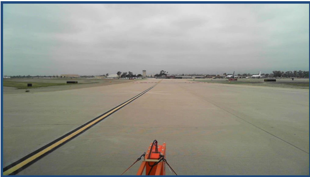
Figure F.13. Taxiway K Representative Pavement Condition (Sta. 5+75)
