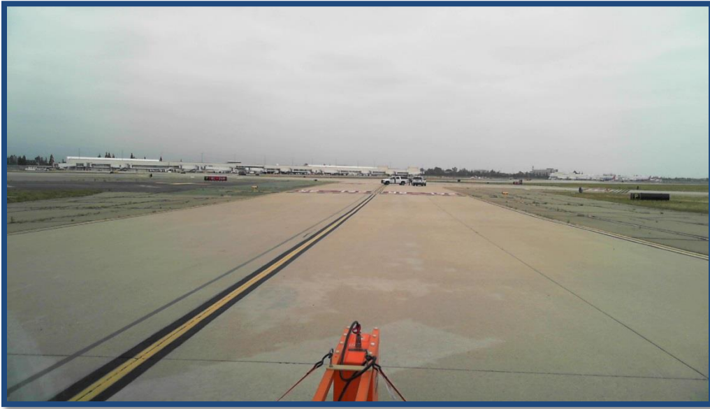
Figure F.16. Taxiway P Representative Pavement Condition (Sta. 6+50)
