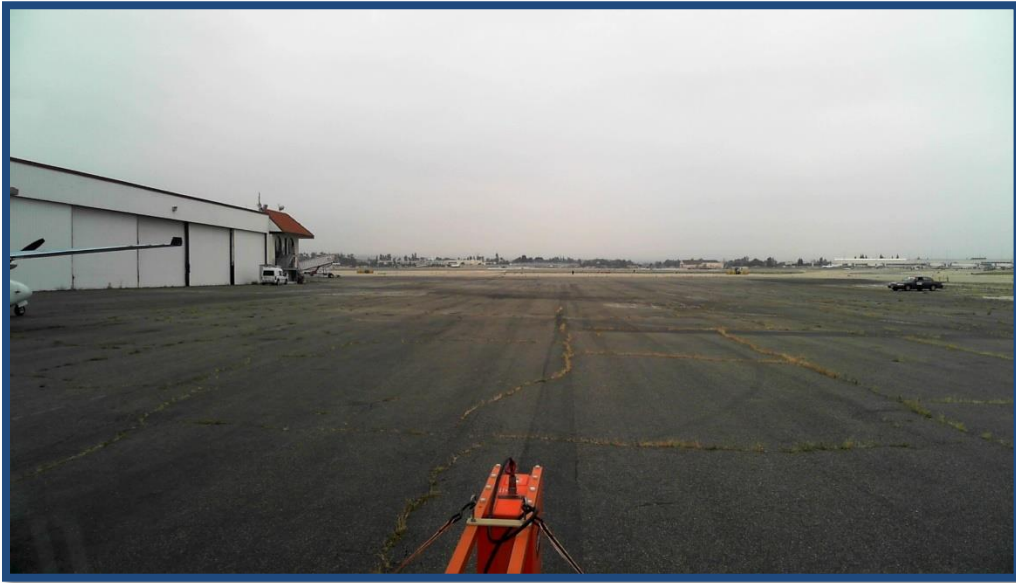
Figure F.36. Atlantic Terminal Apron Representative Pavement Condition (Sta. 3+50)
