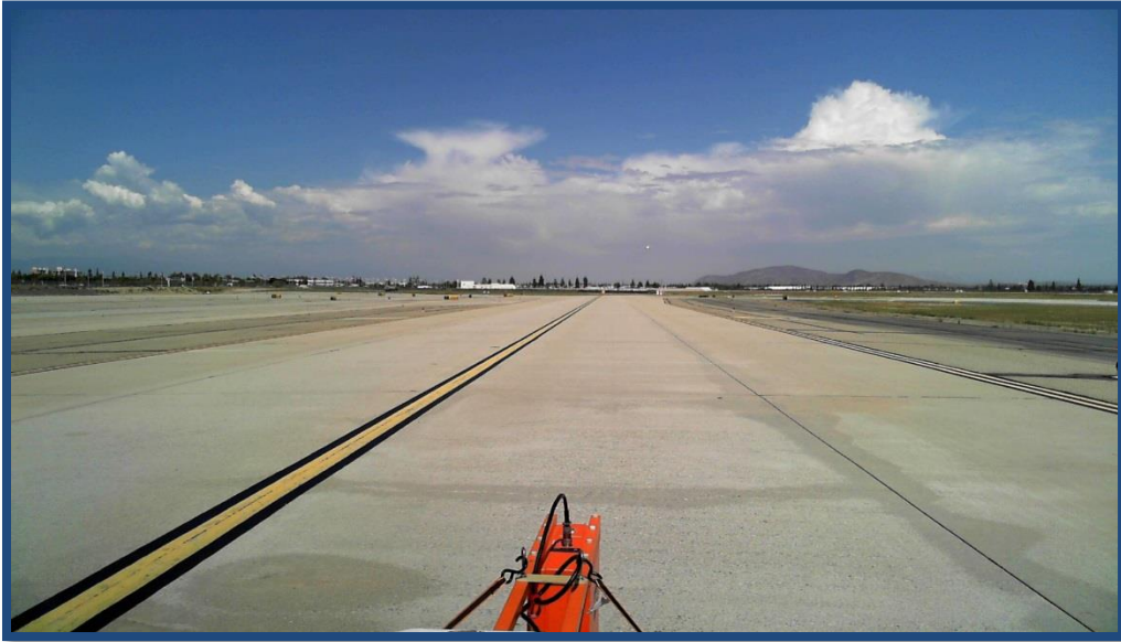
Figure F.4. Taxiway N Representative Pavement Condition (Sta. 110+00)
