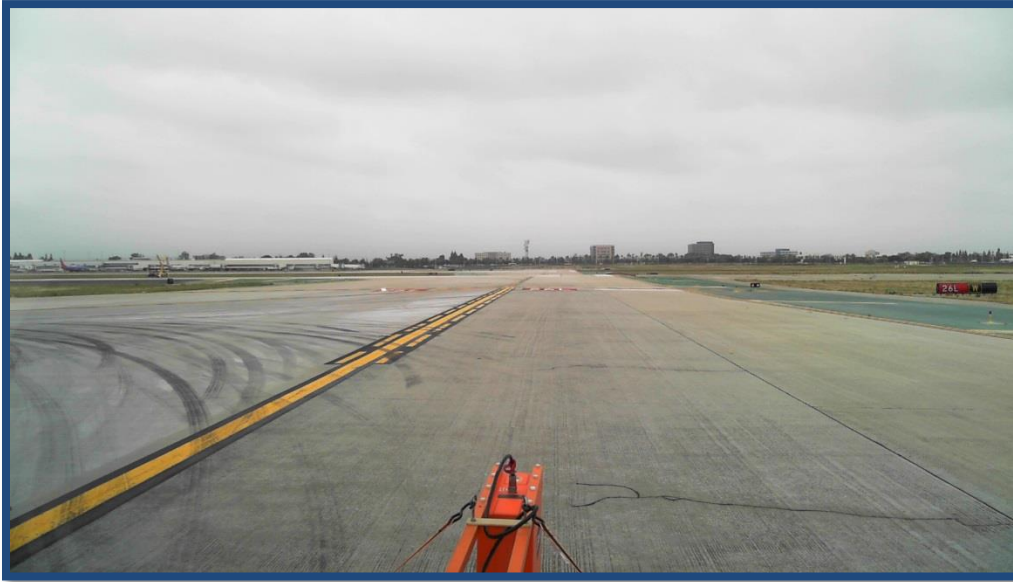
Figure F.28. Taxiway W Representative Pavement Condition (Sta. 4+05)
