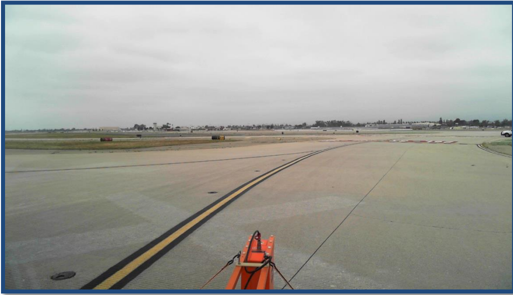
Figure F.18. Taxiway Q Representative Pavement Condition (Sta. 6+30)
