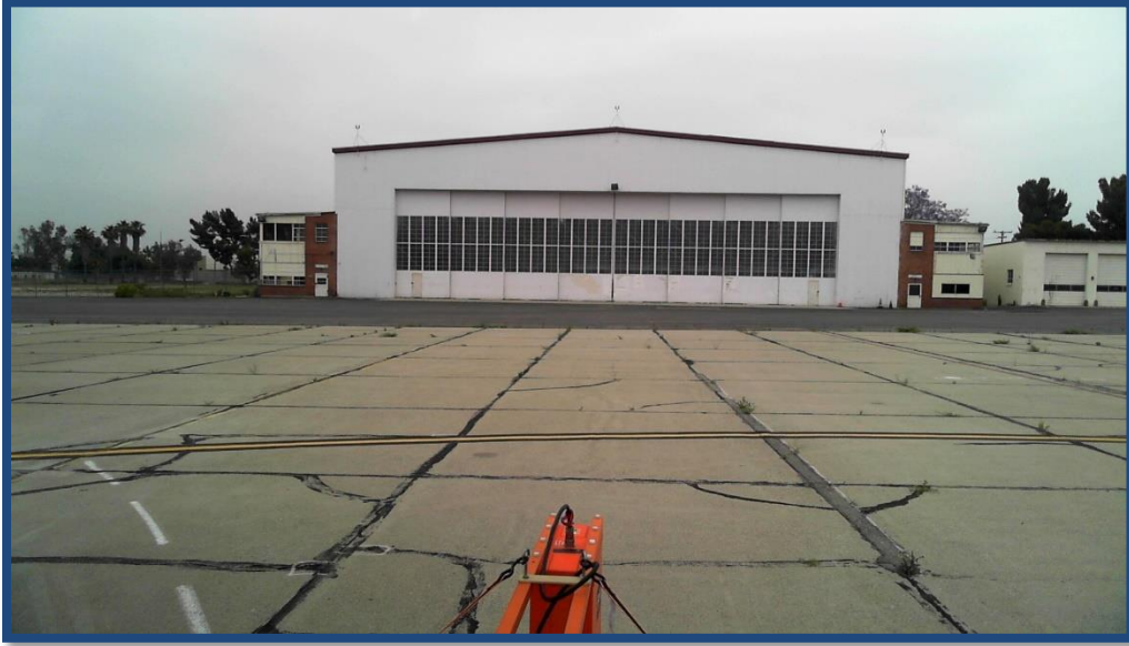
Figure F.38. CSA Terminal Representative Pavement Condition (Sta. 1+50)
