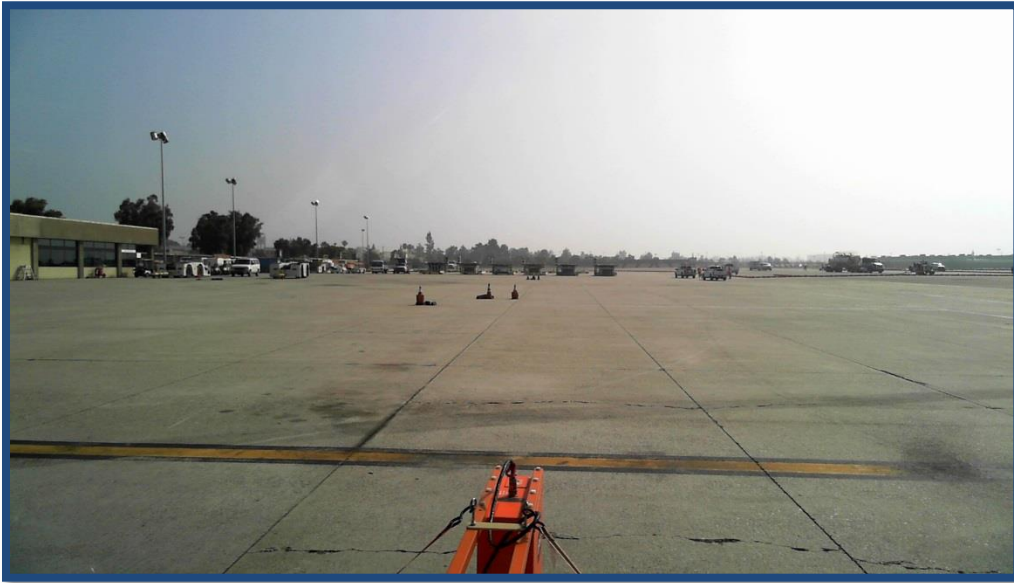
Figure F.34. Terminal 1 Apron Representative Pavement Condition (Sta. 2+08)
