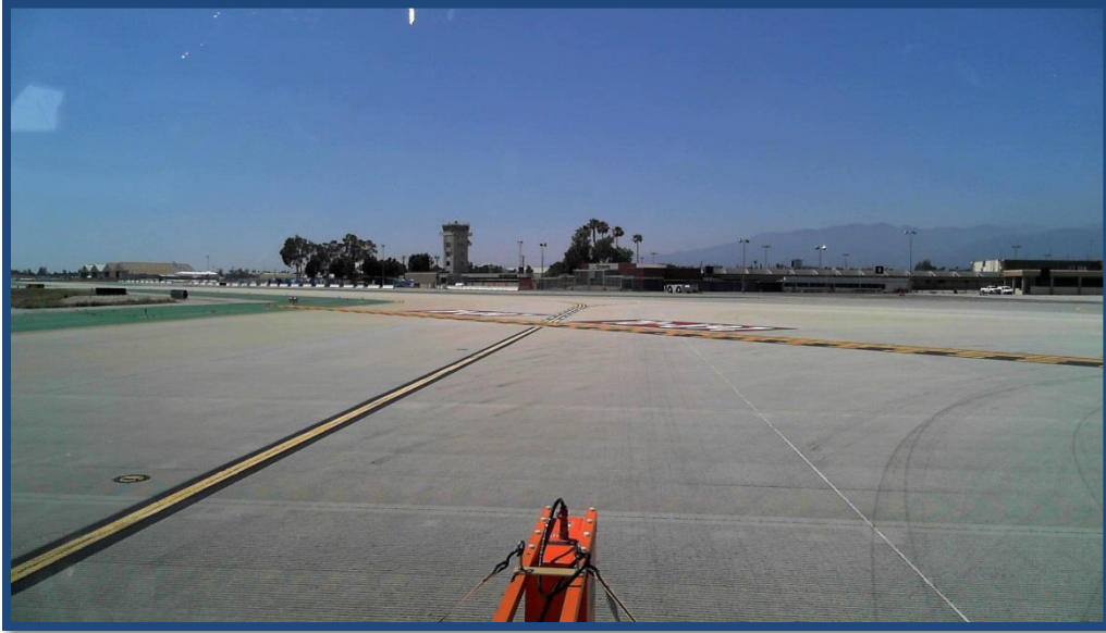
Figure F.14. Taxiway K Representative Pavement Condition (Sta. 7+99)
