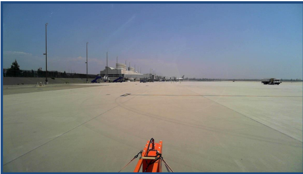
Figure F.35. Terminal 3 Apron Representative Pavement Condition (Sta. 5+50)
