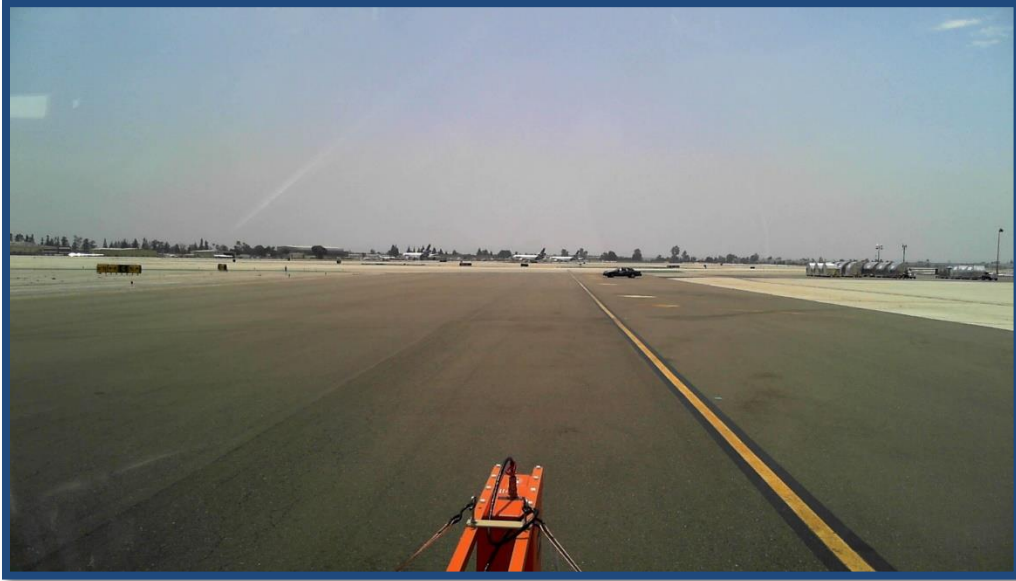
Figure F.40. Taxiway G Representative Pavement Condition (Sta. 1+75)
