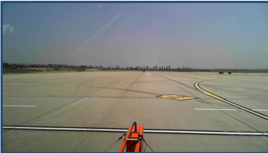
Figure F.43. Taxiway N1 Representative Pavement Condition (Sta. 48+00)
