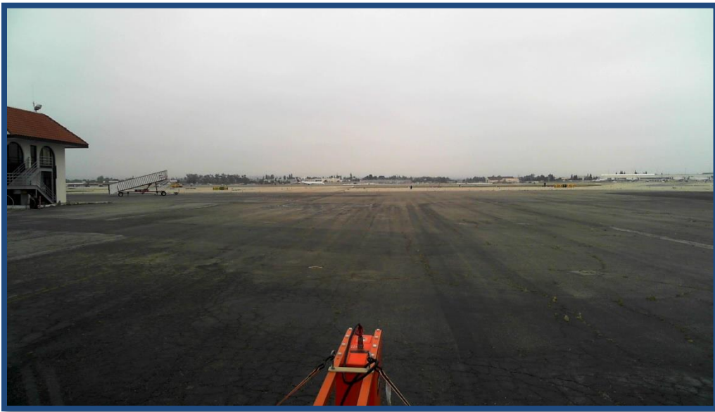
Figure F.37. Atlantic Terminal Apron Representative Pavement Condition (Sta. 5+00)
