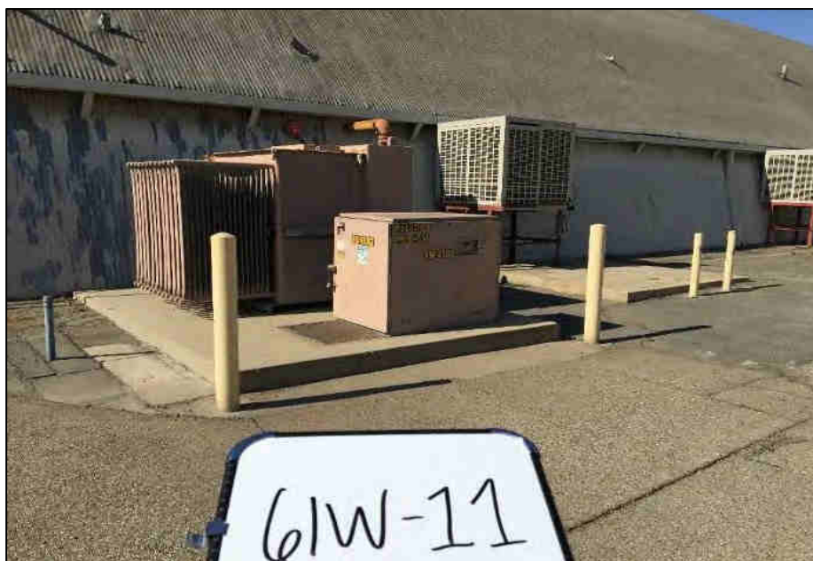
Pad mounted electric box and transformer on eastern corner of hangar 3.
