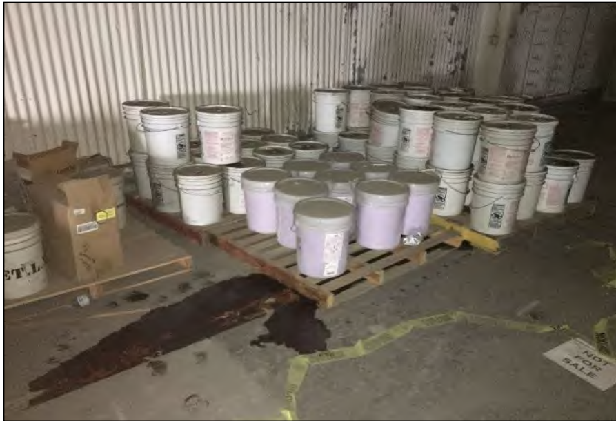
Inside hangar 4 where 5-gallon buckets of AMERX BC Purple K dry were found leaking.
