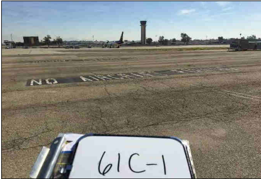
Painted "No Aircraft Parking" sign to the east of the Guardian Jet Center East hangar.
