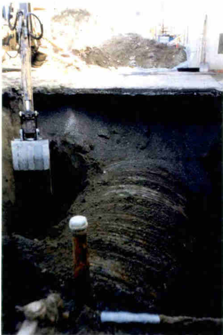
Photo 7. Tank 9 looking toward undermined concrete slab of Tank 10. Note caved gravel backfill from Tank 10. Clean stockpiles in background.
