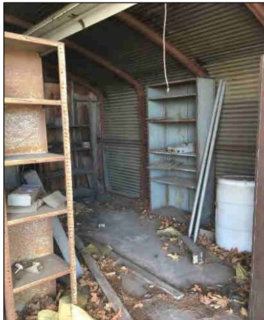
Inside of the shed to the northeast of building #3 where an EA-200 drum is located.
