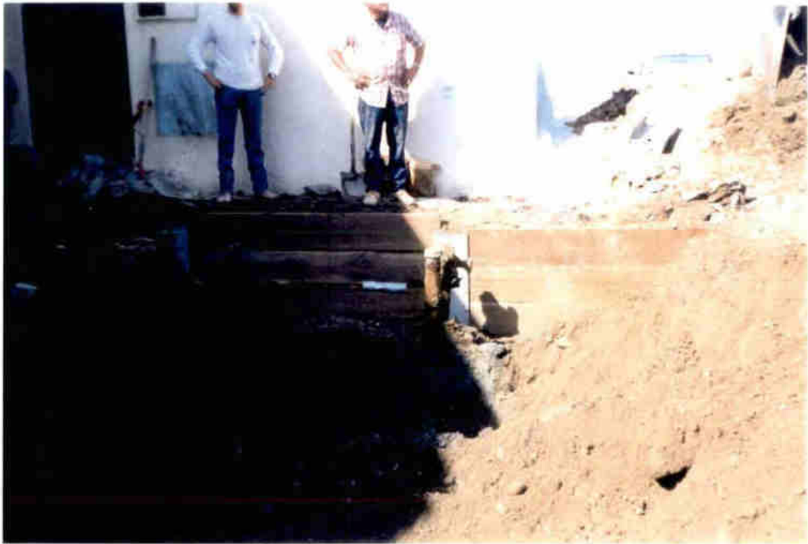
Photo 5. Shoring system for Tank 9. Note bluish-gray soils around fill pipe. Horizontal pipe leading to left is product delivery pipe.
