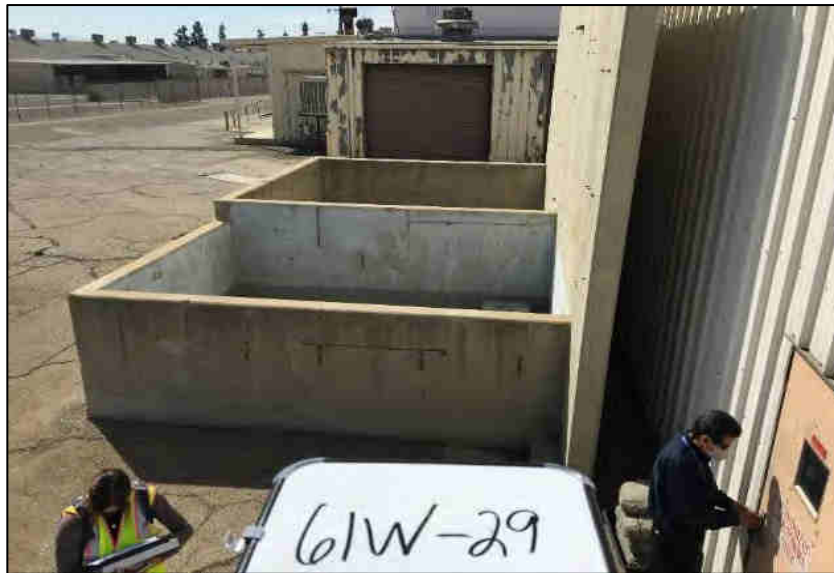
Looking south towards concrete enclosures for former ASTs east of 61W-29 building.
