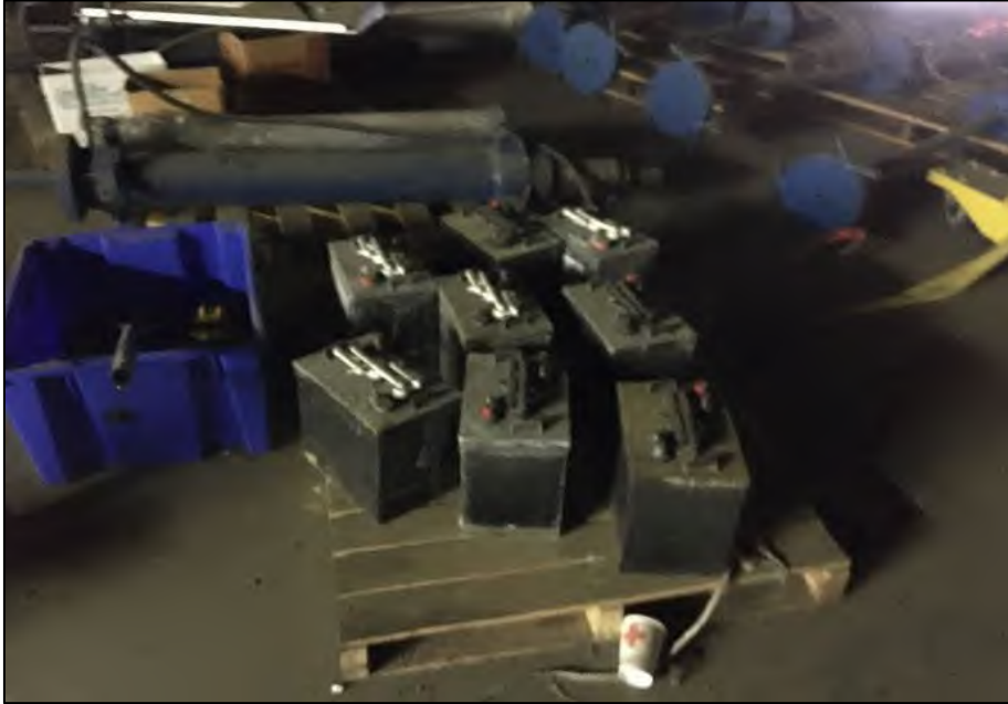
Inside of 61W-32, building #4. Eight batteries.
