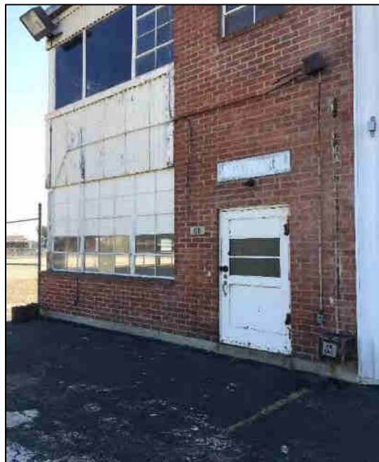
Looking at the maintenance building to the east of the former CANG hangar.
