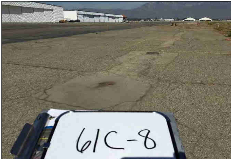
Long trench coming from the drain inlet that could be a possible former clarifier location.
