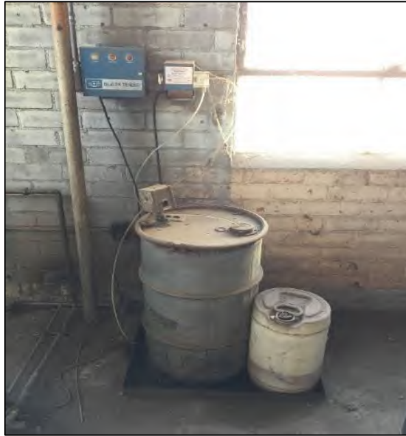
Inside of the boiler room.
