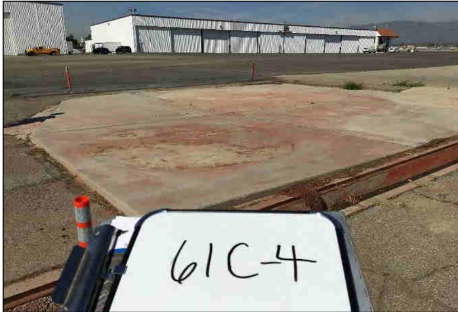
Former wash rack to the east of the Guardian Jet Center hangars with red staining. An outline of former AST is also visible.
