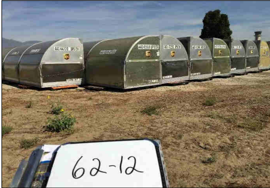
UPS pods on top of a concrete pad that used to be a former maintenance shop.
