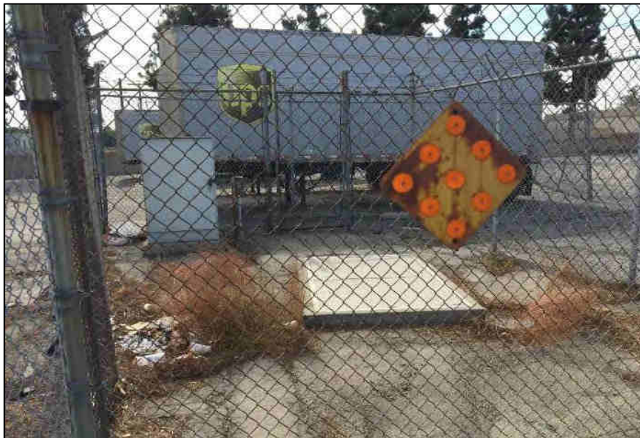
Looking east at the General Telephone underground utility.
