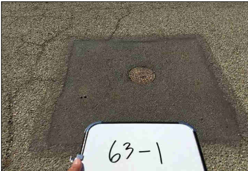
Southern California Gas lid surrounded by an asphalt patch located in the southeastern portion of Parcel 63.
