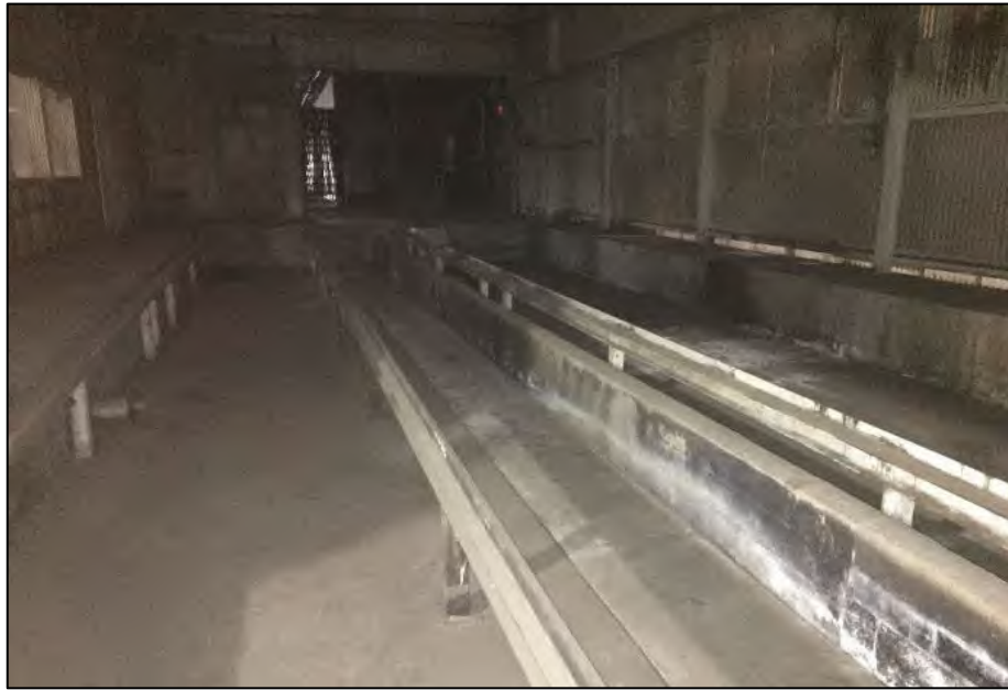
The northeast corner of hangar 1 where a drainage sump with missing grates is located.
