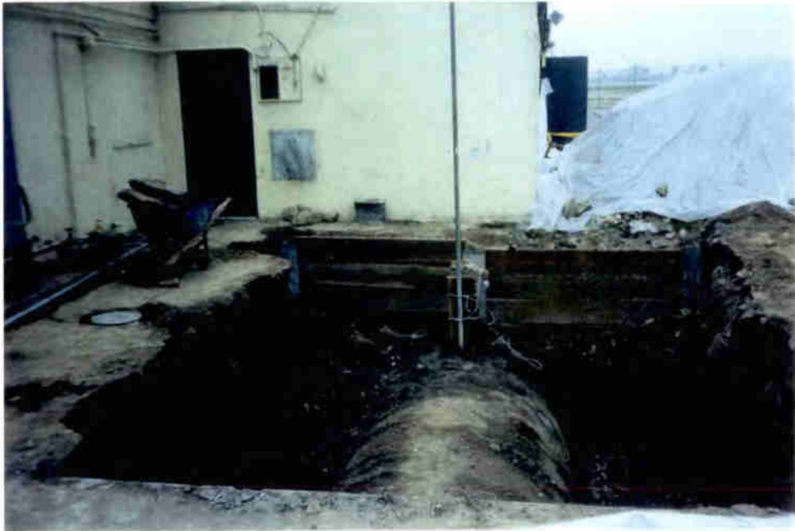
Photo 9. Tank 9 excavated with temporary vent installed. Monitoring Well MW-10 to left. Note Calibration Fluid affected stockpile in right background, covered with plastic sheeting to reduce vapor emissions.
