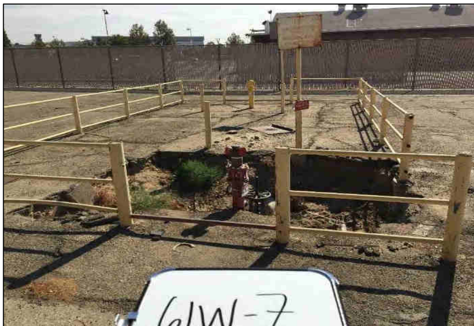
Facing west where fire sprinkler piping and an excavation pit is located.
