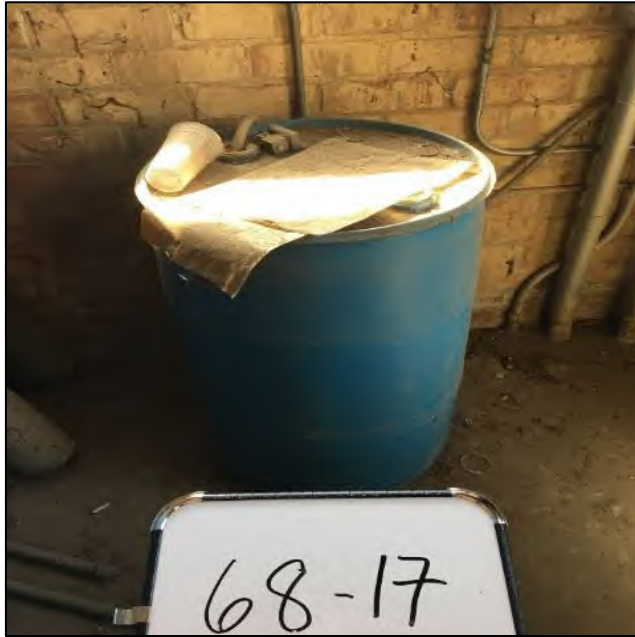
Inside of the boiler room.
