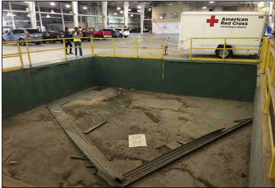
Sunken pit with drain in the northwest corner of the administration building/hangar 2.
