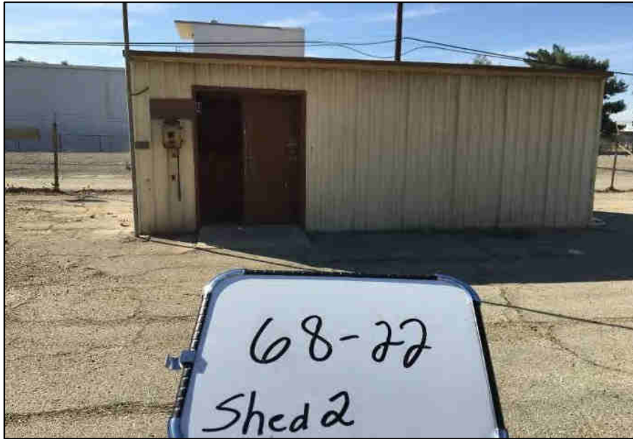
Looking south towards the shed in the southwest corner of the maintenance yard.
