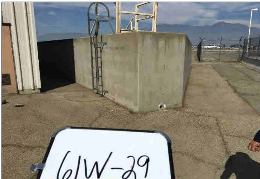
Looking north at concrete enclosure for former ASTs north of 61W-29 building.
