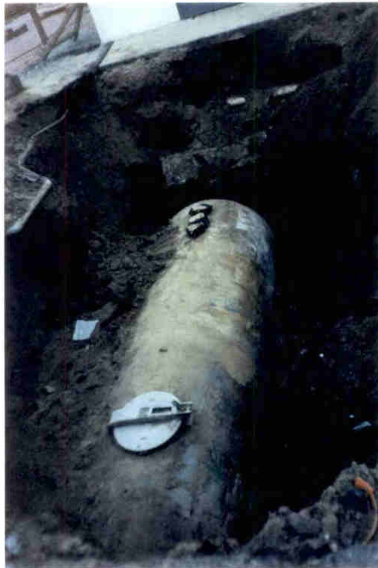
Photo 8. Tank 11 excavated. Note exposed water main to left; telephone duct top center; and concrete slab beneath duct.
