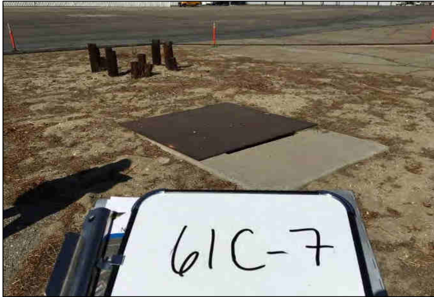
Steel lid utility vault east of the Guardian hangars.
