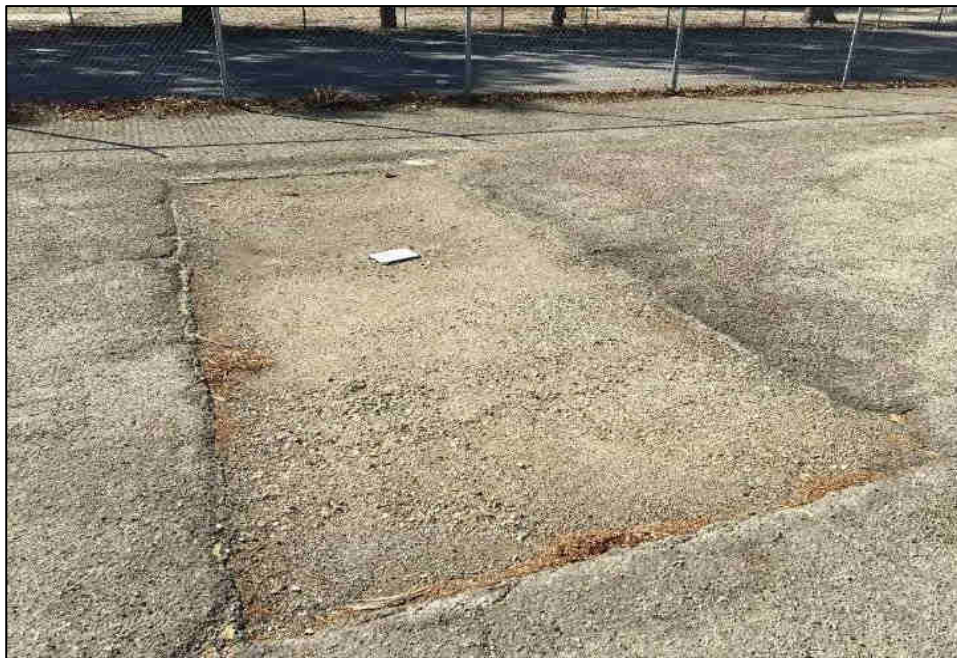
Rectangular back filled area with tie downs located south of the former National Guard Motorcycle shop.
