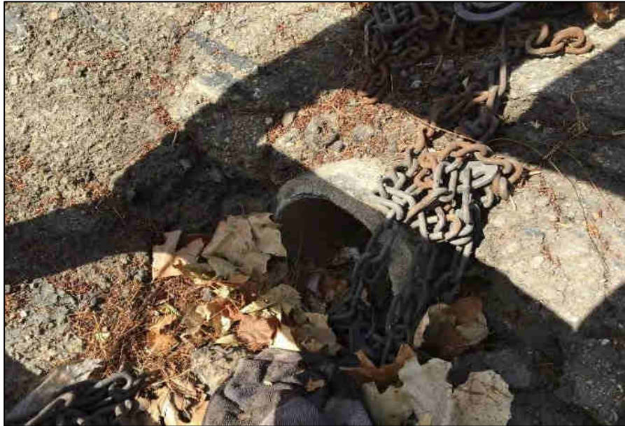
Drain inlet located in the middle of the parking lot next to hangar 4.
