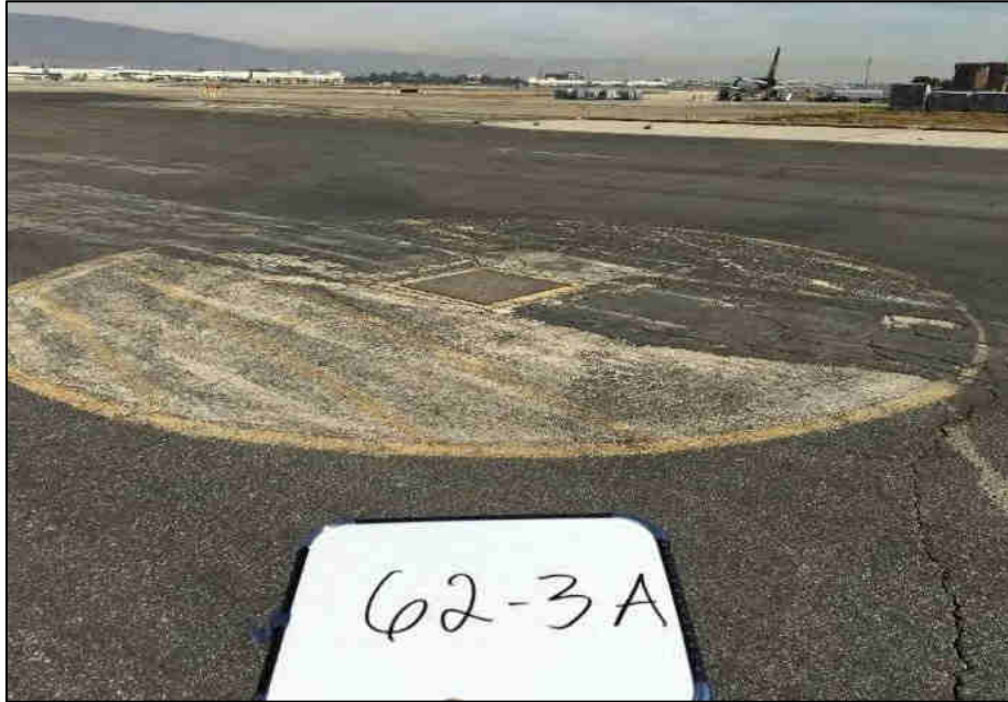
Helicopter pad with possible destroyed inlet to the east of the Guardian East hangar.
