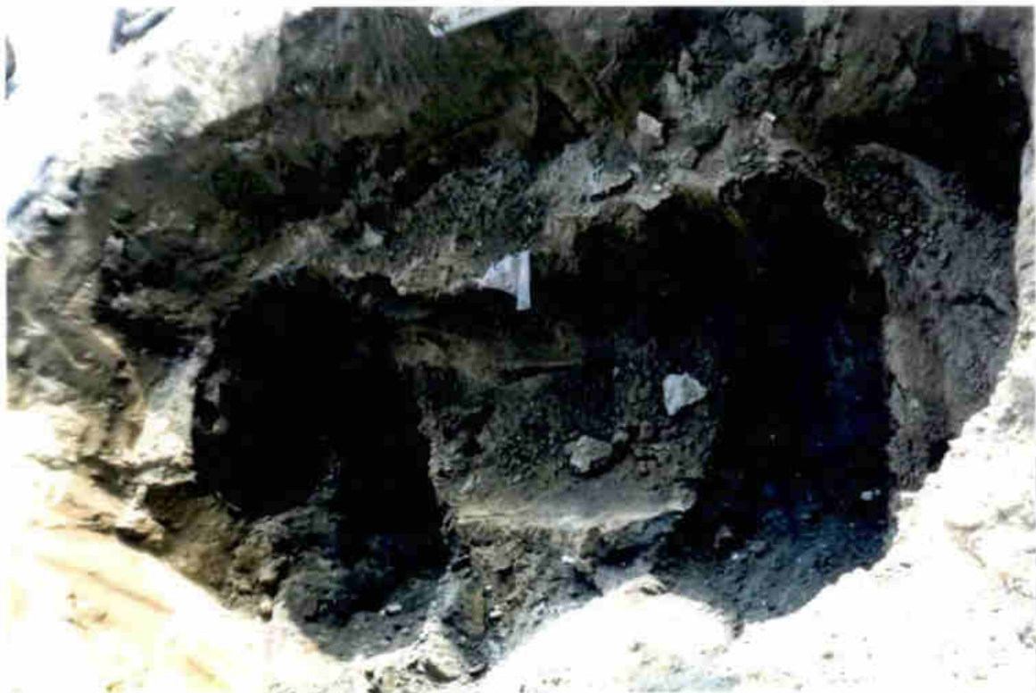
Photo 12. Tank 11 excavation. T-1 Sample locations to right; T-2 Sample locations to left. Jet A Fuel affected soils, stained bluish-gray, were subsequently removed.
