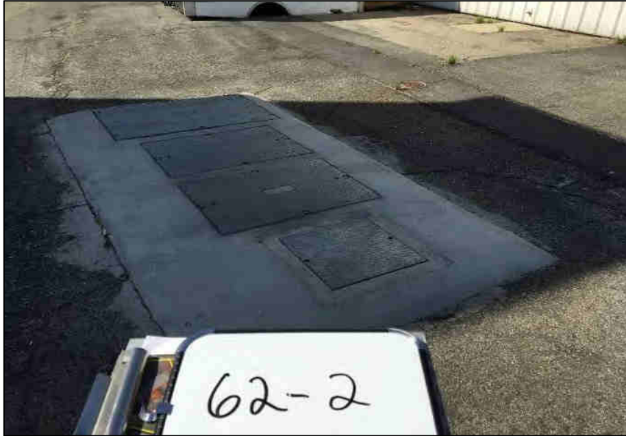
Four stage clarifier in between the Guardian hangars.
