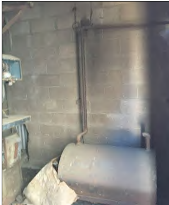
Looking inside at a possible AST associated with the HVAC system at 61W-1.
