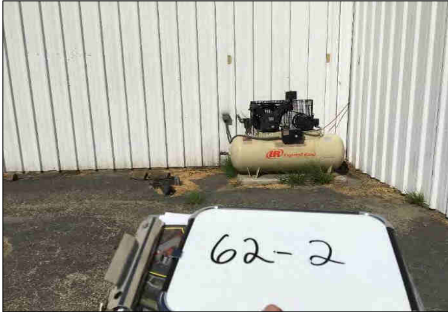
Air compressor tank in the southeastern corner of the Guardian Jet Center southern hangar.
