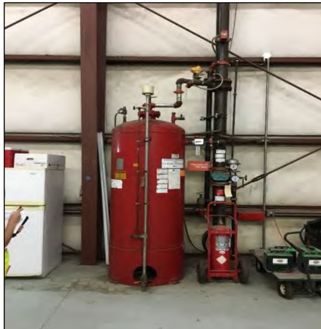
AFFF suppression system inside the Guardian Center southern hangar.
