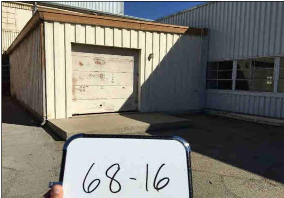
Facing north towards the ancillary hangar building west of the motorcycle shop.
