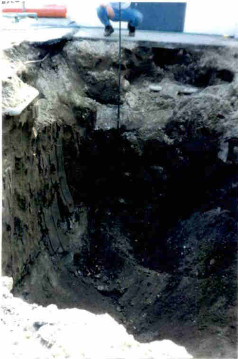
Photo 13. Tank 11 excavation before backfill. Black stick measures 10 feet to surface. Total excavation depth measured approximately 14 feet from surface.
