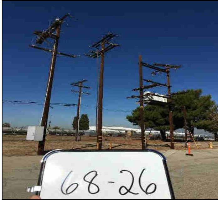
Powerlines at the southwest corner of the former National Guard lease area.
