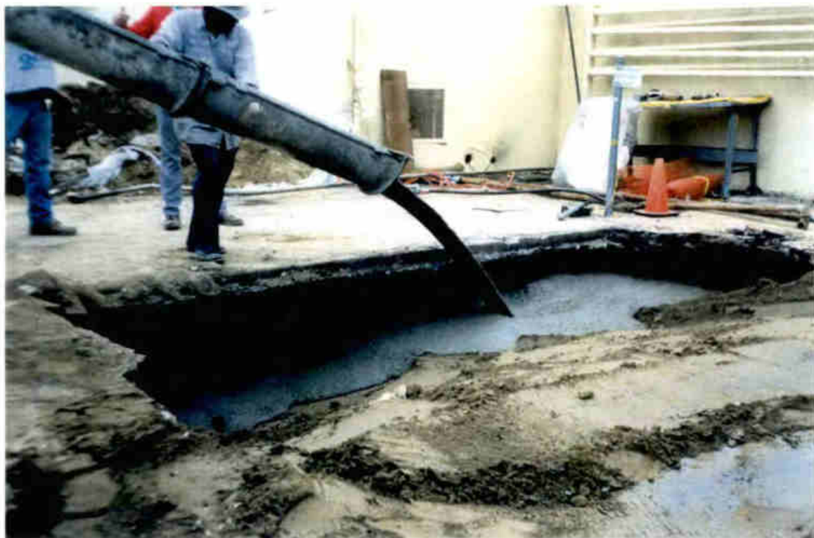
Photo 10. Placing control density backfill slurry beneath undermined Tank 10 concrete slab. Tank 9 was backfilled with clean soil and ramped towards Tank 10 to improve flow of slurry beneath slab.
