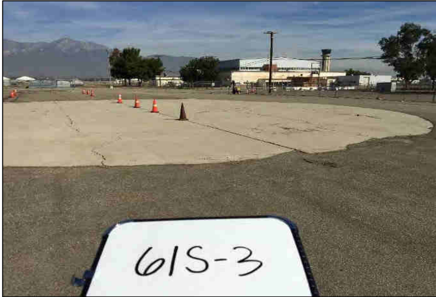
Circular concrete patch on the west side of the southern portion of Parcel 61.
