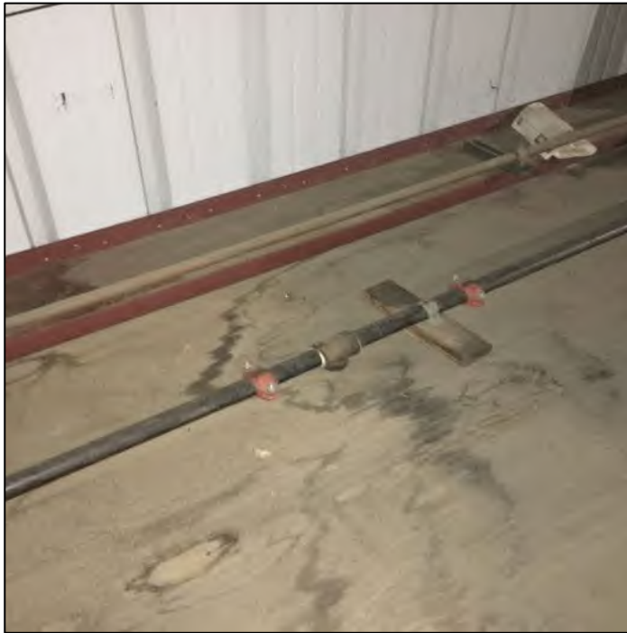
Staining from possible leaking AFFF piping upstairs.
