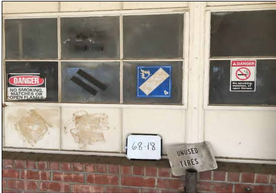
Hazardous placard located on the glass north of the awning.
