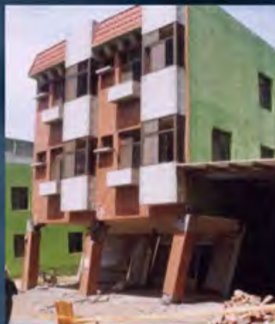
1999 Chi-Chi (Taiwan) Earthquake
