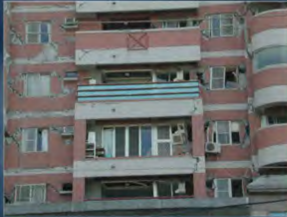
1999 Chi-Chi (Taiwan) Earthquake
